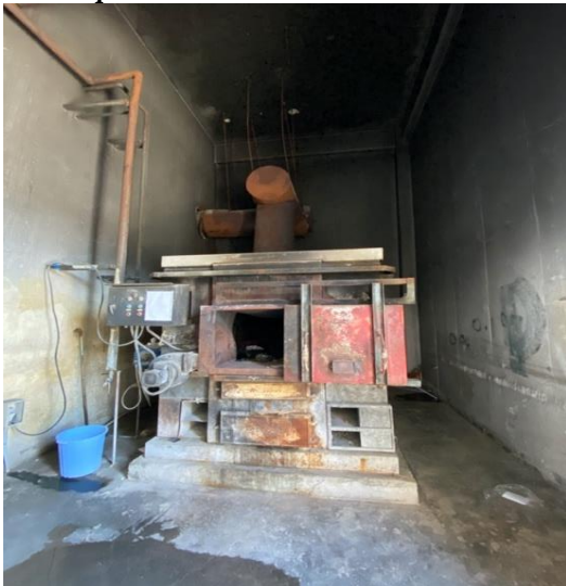
Fig. (20): Incineration treatment plant of Azadi hospital
