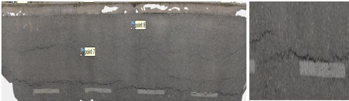
Fig. (14): a- Orthomosaic of the street distresses obtained from a side position camera b- A zoomed-in view of the crack section
