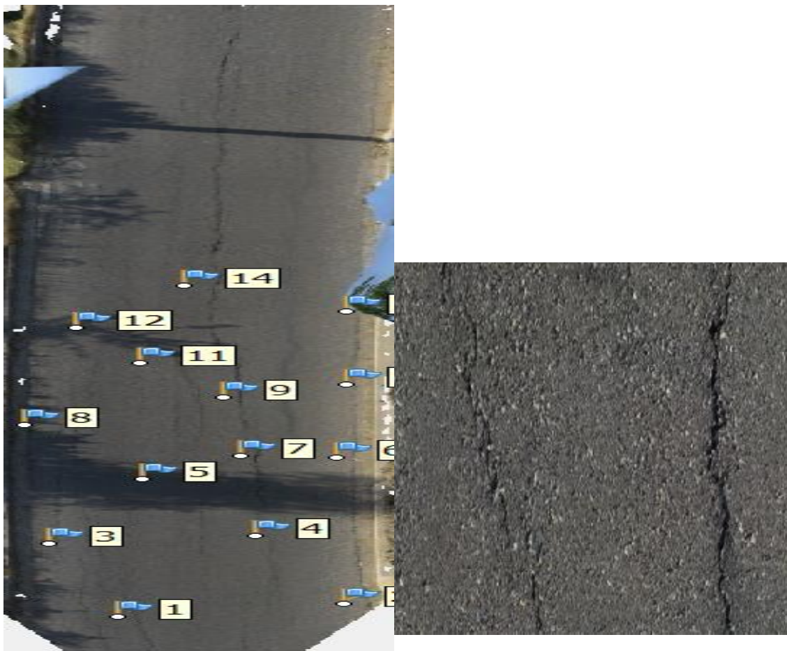
Fig. (17): a-Orthomosaic of the street distresses obtained from a front position camera
