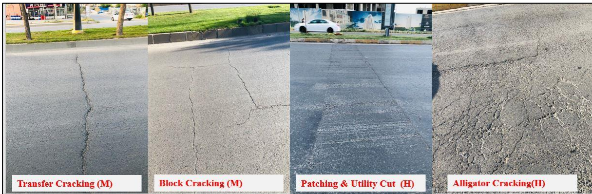
Fig. (2): Samples of pavement distresses in the case study
