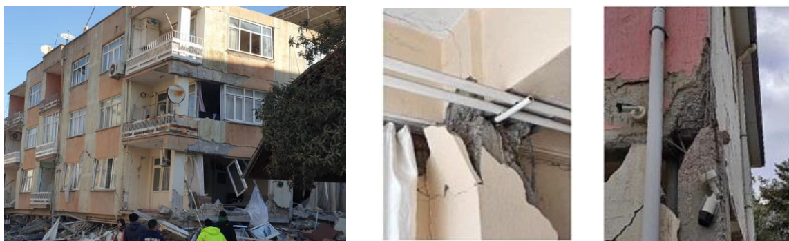
Fig.( 5):- collapse and damage due to strong beam and weak column (Mertol et al., 2023; OZTURK et al., 2023).
