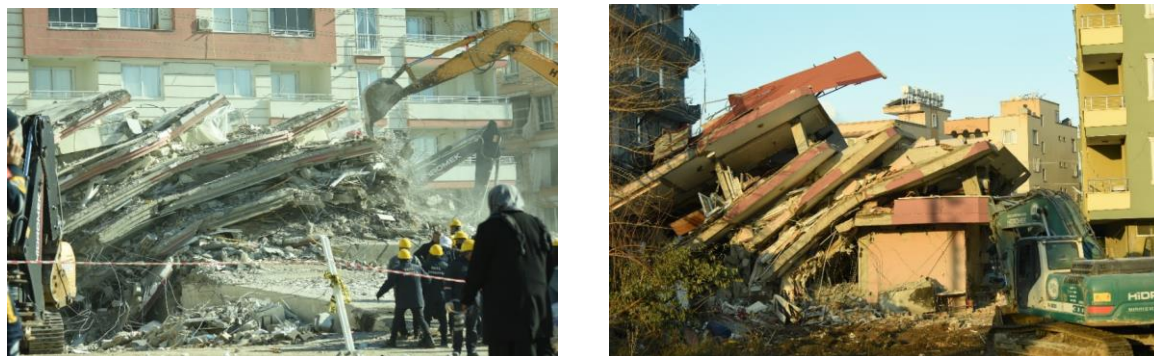
Fig.( 17):- Damage to the load-bearing system with complete building collapse (Lekkas et al., 2023).
