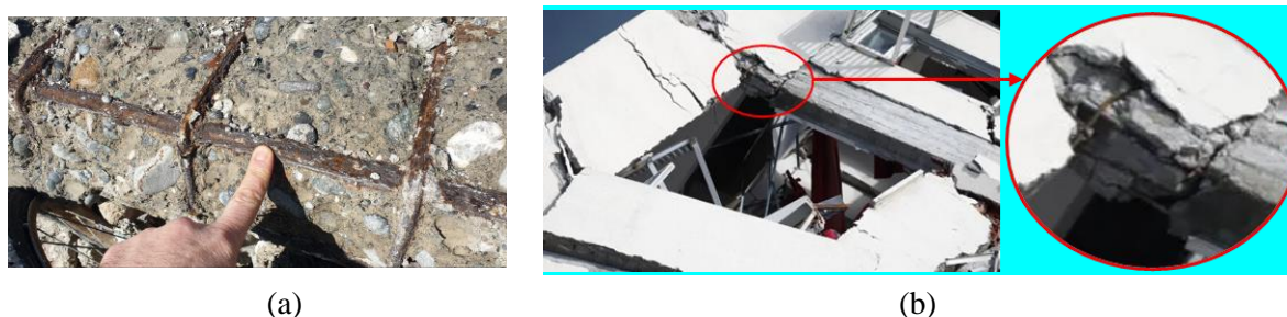
Fig.( 4):- Corrosion in: (a) longitudinal and transverse reinforcements (Mertol et al., 2023); and (b) beam-column connection (Alhawamdeh et al., 2023).
