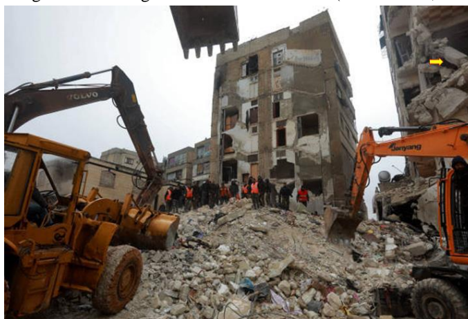
Fig.( 6):- Extensively damaged RC columns (marked by arrows) in a building adjacent to ruins of a collapsed building in Hama (Alhawamdeh et al., 2023).
