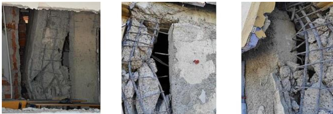
Fig.( 14):- Earthquake-damage to a retrofitted high school building in Kahramanmaraş (OZTURK et al., 2023).
