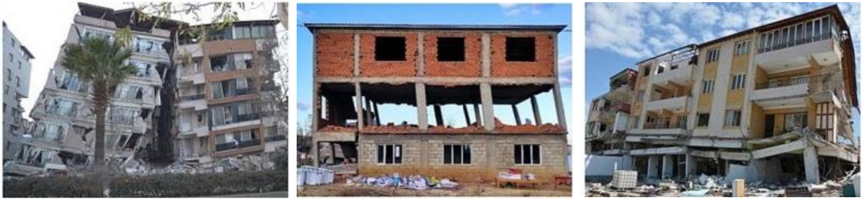
Fig.( 9):- Collapses resulting from soft or weak stories in RC buildings (OZTURK et al., 2023).
