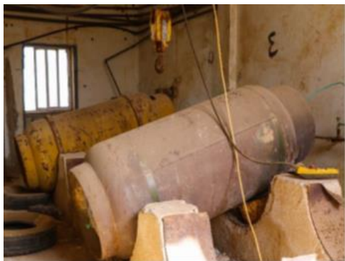
Fig.( 4): -Chlorine gas cylinders
