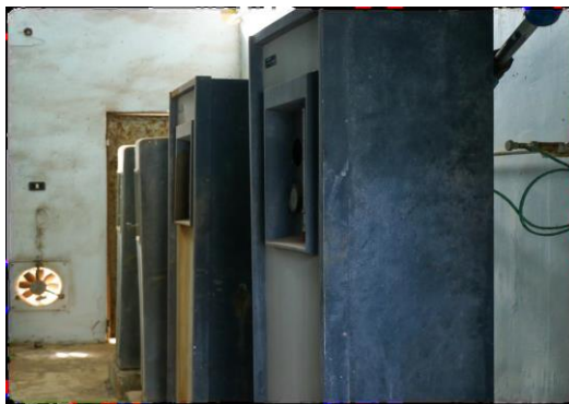
Fig.( 3): -Primary chlorine gas devices
