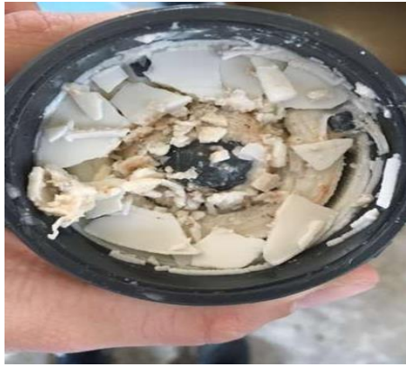
Fig.( 6): -Damage to pipes due to the use of gas
