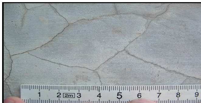
Fig.( 11):- Cracking crack [29].
