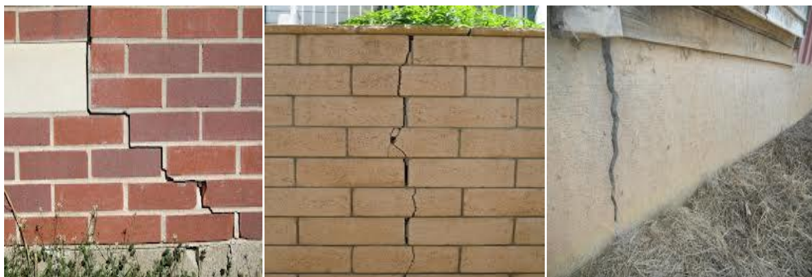
Fig.( 5):- Cracking due to movement or settling of the ground [24].
