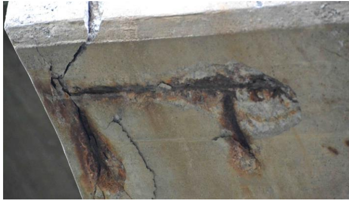
Fig.( 6):- Concrete crack due to reinforcing bar corrosion [26].
