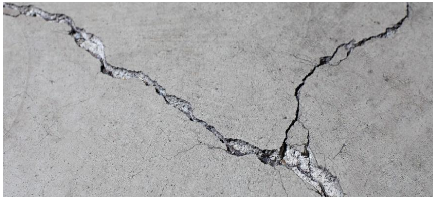
Fig.( 7):- Sulphate attack cracks [1]
