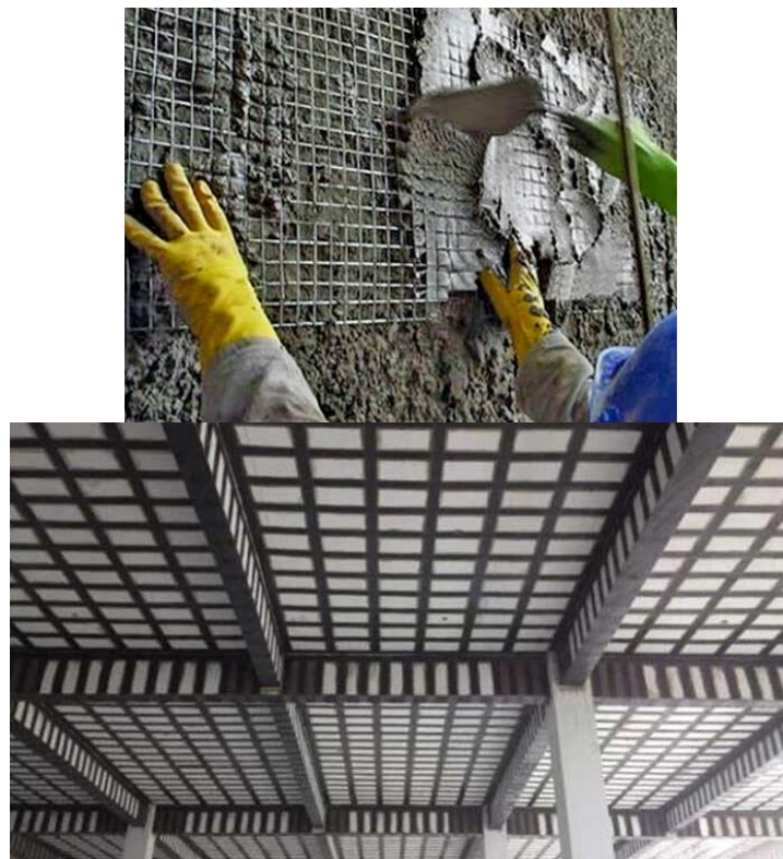
Fig.( 3):- Mesh steel reinforcement [18].
