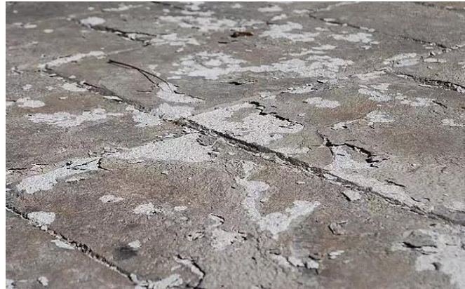
Fig.( 9):- Freezing and thawing cracks [27].
