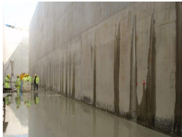
Fig.( 4):- Early thermal cracks [17]
