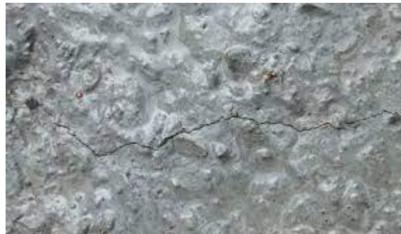
Fig.( 10):-: Autogenous Shrinkage Cracks [28].
