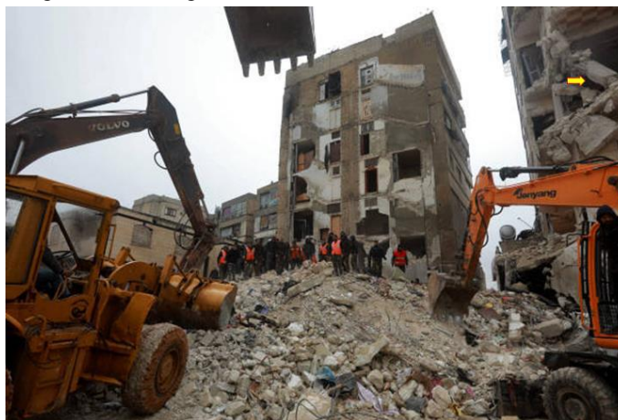
Fig.( 6):- Extensively damaged RC columns (marked by arrows) in a building adjacent to ruins of a collapsed building in Hama (Alhawamdeh et al., 2023).
