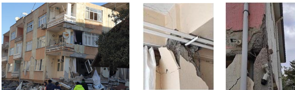
Fig.( 5):- collapse and damage due to strong beam and weak column (Mertol et al., 2023; OZTURK et al., 2023).
