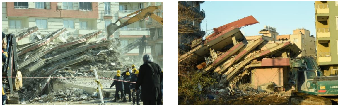
Fig.( 17):- Damage to the load-bearing system with complete building collapse (Lekkas et al., 2023).
