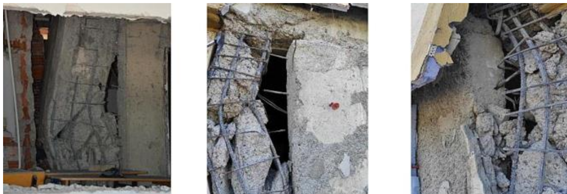
Fig.( 14):- Earthquake-damage to a retrofitted high school building in Kahramanmaraş (OZTURK et al., 2023).
