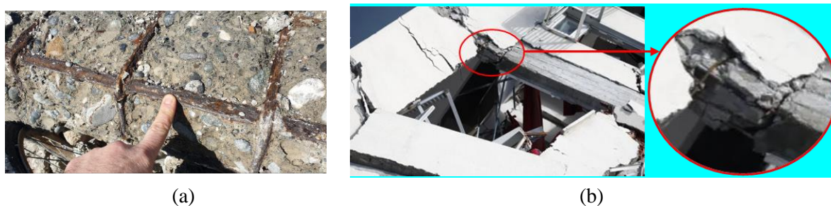
Fig.( 4):- Corrosion in: (a) longitudinal and transverse reinforcements (Mertol et al., 2023); and (b) beam-column connection (Alhawamdeh et al., 2023).
