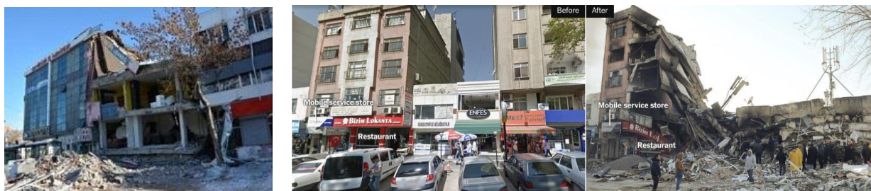
Fig.( 15):- Damage and collapses of buildings due to pounding effects (Alhawamdeh et al., 2023; OZTURK et al., 2023).
