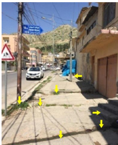
Fig. (8): Sidewalk with poor concrete surface (Source: the authors)
