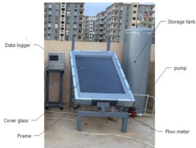
Figure (2) solar water heating system
