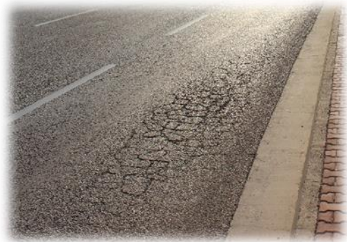
Fig. (2): Fatigue Cracking
