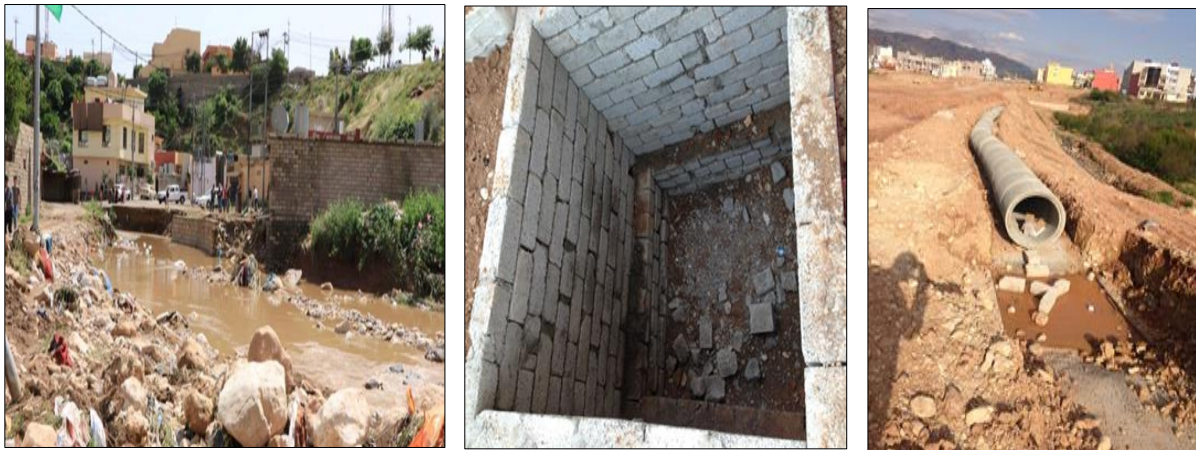
Fig. (4) Hishkarow river in Duhok city, a non-regulated Septic tank, and New sewer line under construction
