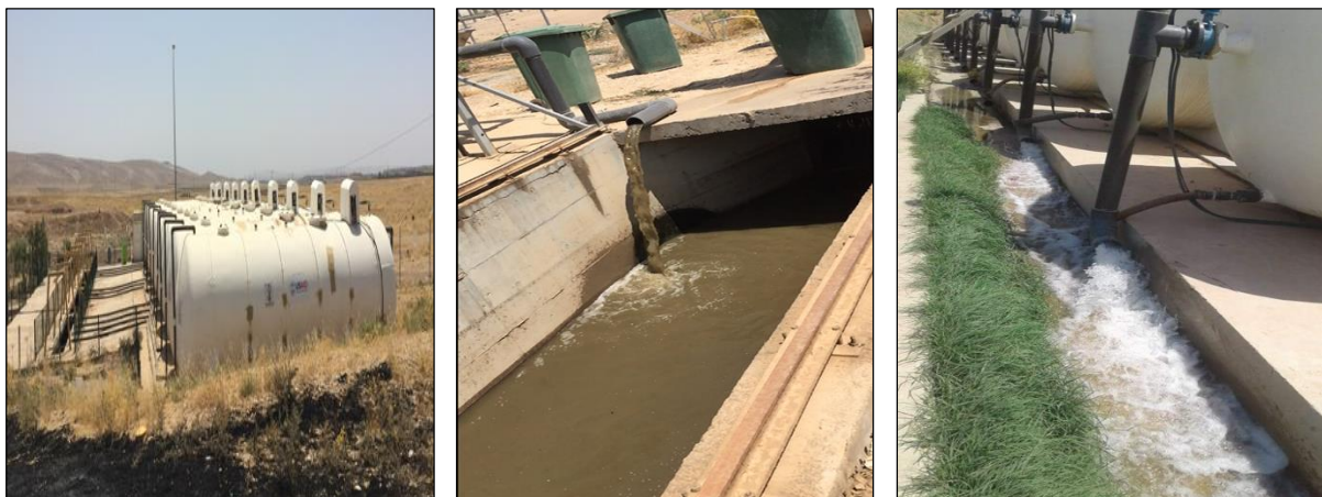
Fig. (7): Package sewage treatment plant of Sharia IDPs camp
