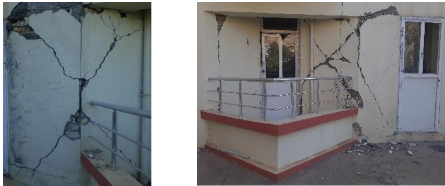
Fig. (25): Diagonal cracks in the infill walls
