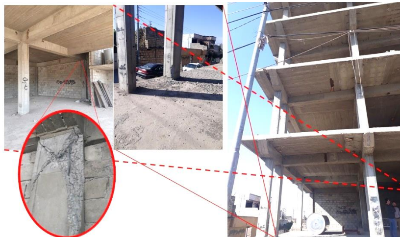
Fig. (5): Damage in a column of a 7-story reinforced concrete building in Halabjah
