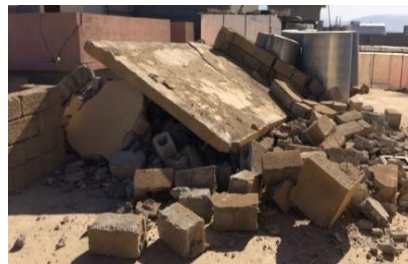
Fig. (28): Collapse of the penthouse
