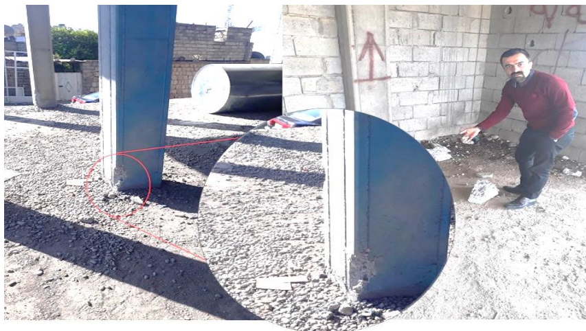
Fig. (6): Easily crushing the concrete by one of the authors as a sign of very weak concrete
