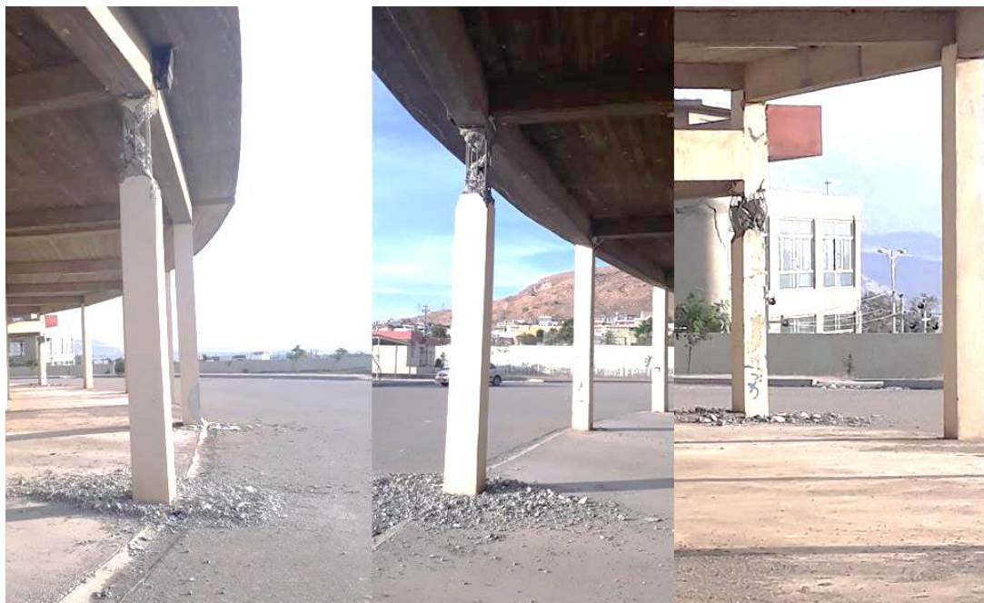
Fig. (21): Hinging in columns at exterior supports
