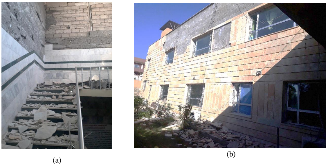
Fig. (26) Finishing material state in the Darbandikhan general hospital (a) Falling off of the tiles inside (b) Hilan stone falling outside.
