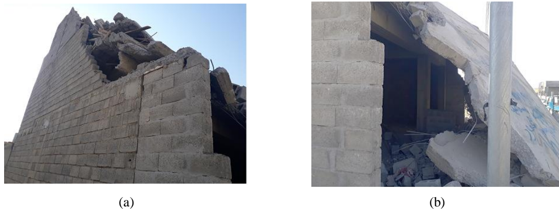
Fig. (16): (a) Rotation of at the base of the third floor (b) A collapsed circular column
