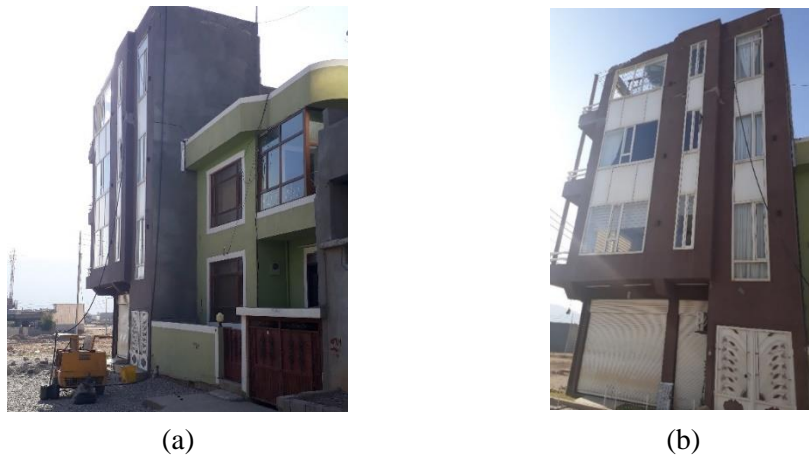
Fig. (24): Rotation of a frame building in Darbandikhan (a) Isometric view of the building showing its back (b) Side view of the building
