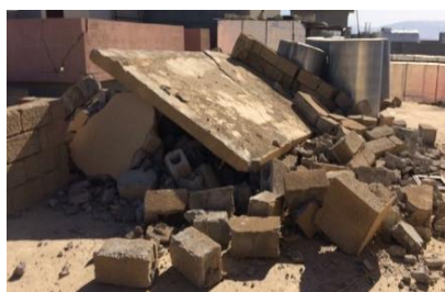
Fig. (28): Collapse of the penthouse
