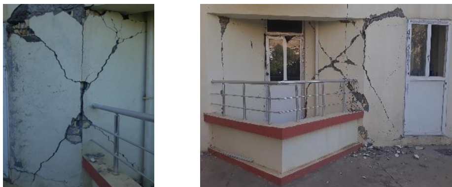
Fig. (25): Diagonal cracks in the infill walls
