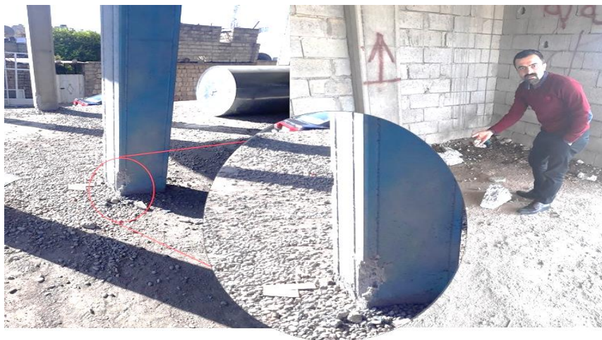
Fig. (6): Easily crushing the concrete by one of the authors as a sign of very weak concrete
