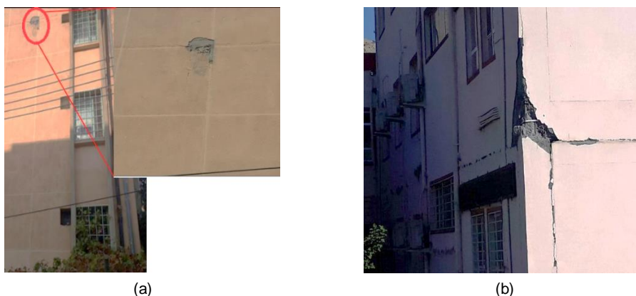
Fig. (27): Concrete spalling in the joints in frame buildings (a) seven-storey residential building in Halabjah (b) Municipality building of Darbandikhan
