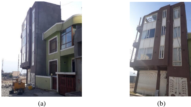
Fig. (24): Rotation of a frame building in Darbandikhan (a) Isometric view of the building showing its back (b) Side view of the building
