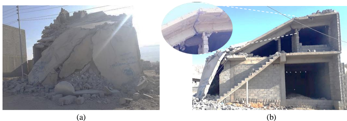
Fig. (15): (a) Front view of a collapsed three-story hybrid building (b) Side view of the same building
