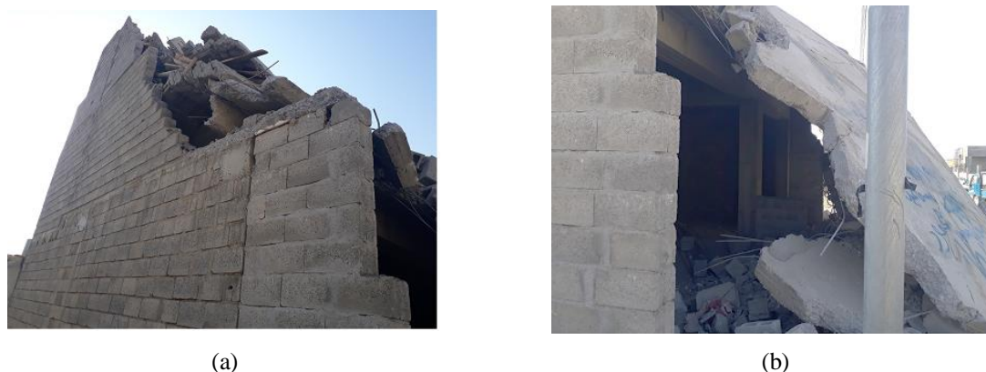
Fig. (16): (a) Rotation of at the base of the third floor (b) A collapsed circular column
