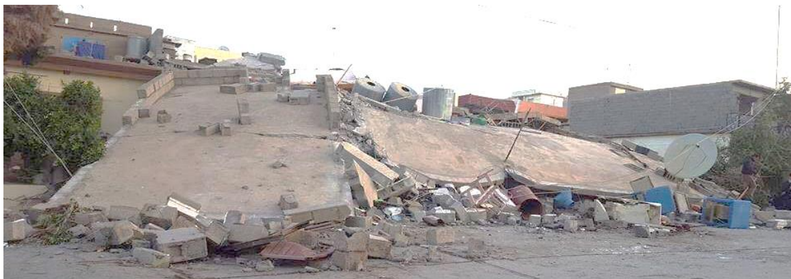
Figure 9. Collapse of a three-story Building using Hybrid system of (R.C Frame- Masonry) (front view)
