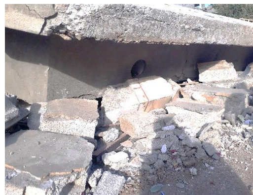
Fig. (11): the scale of the lintel compared to a 40 cm concrete block
