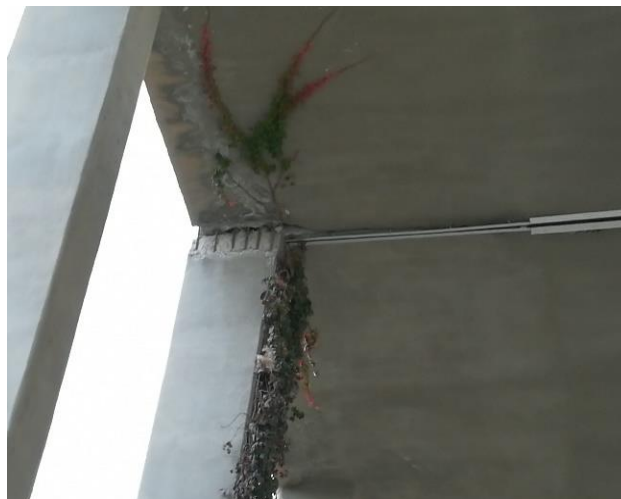
Fig. (8): Pounding effect between two columns in the Children Hospital in Halabjah
