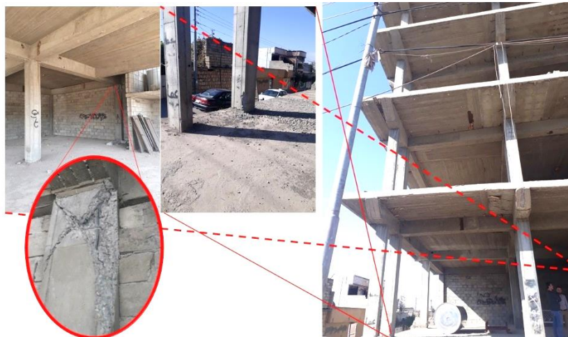
Fig. (5): Damage in a column of a 7-story reinforced concrete building in Halabjah
