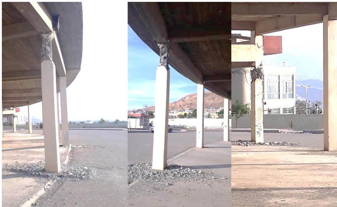
Fig. (21): Hinging in columns at exterior supports
