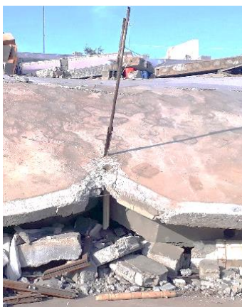
Fig. (10): Large R.C lintels of depth of more than one meter in front of the house
